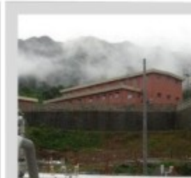
Sibayak Geothermal Power Plant in Indonesia
